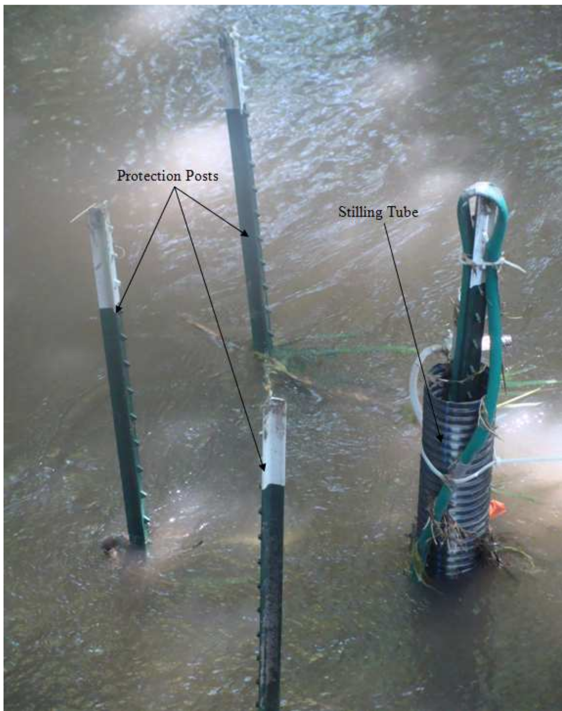
Figure 4.2. Installed pressure transducer
